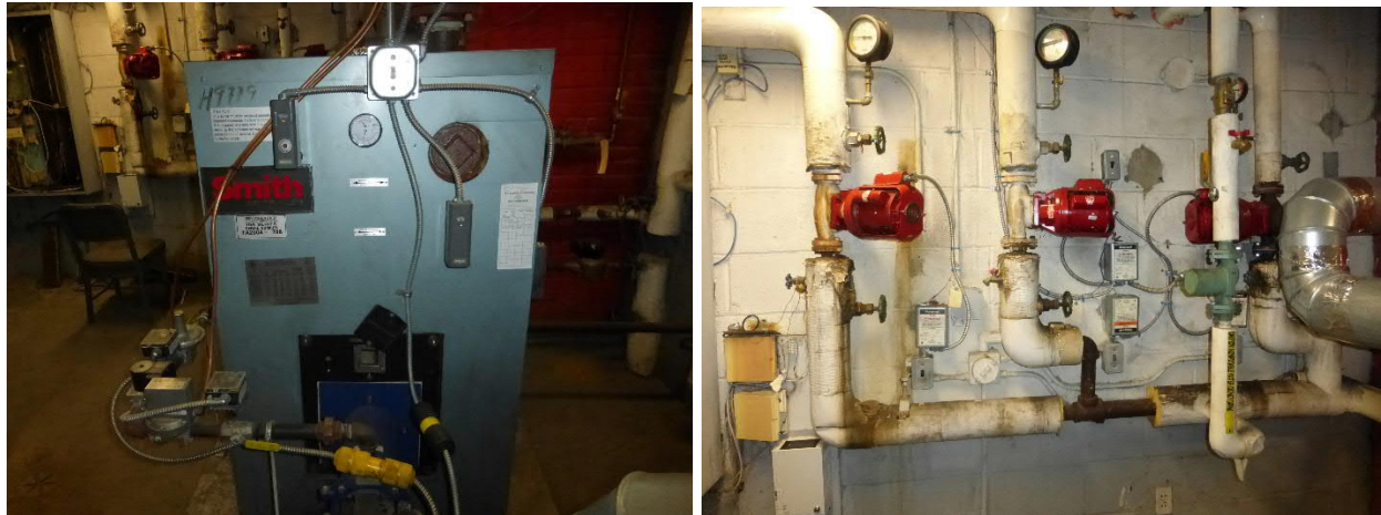
Figure 2 – Boiler and Pumps
