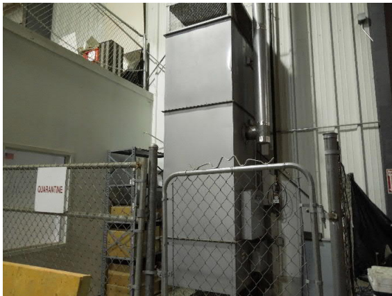
Figure 2 – Building 600 Air Turnover Unit
