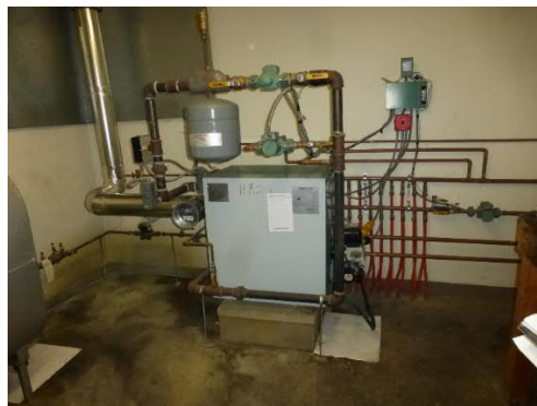
Figure 3. Building 123 Fuel Oil Fired Boiler, Typical of Three
