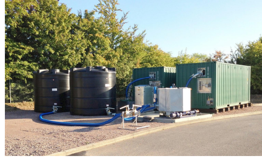
Figure 8-1. Anaerobic Biogas Generator
