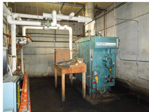
Figure 2. Building 96 Boiler Room
