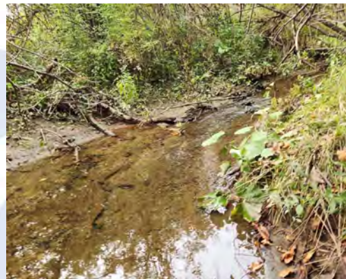
Example of degradation in Reach MB 2A.
